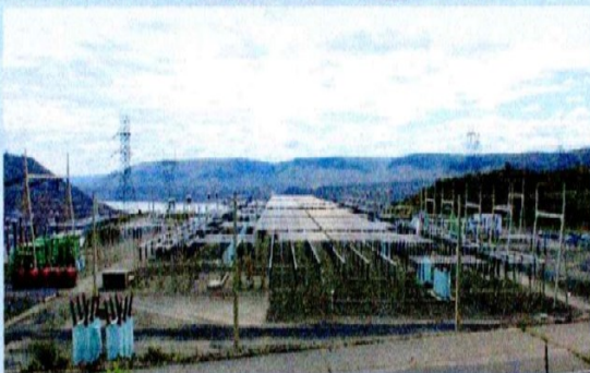
500 kV switchyard, Grand Coulee Dam
