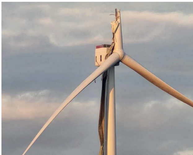
Vineyard Wind turbine blade that was damaged on July 13 captured by a New Bedford commercial fisherman. Photo courtesy of Anthony Seiger
